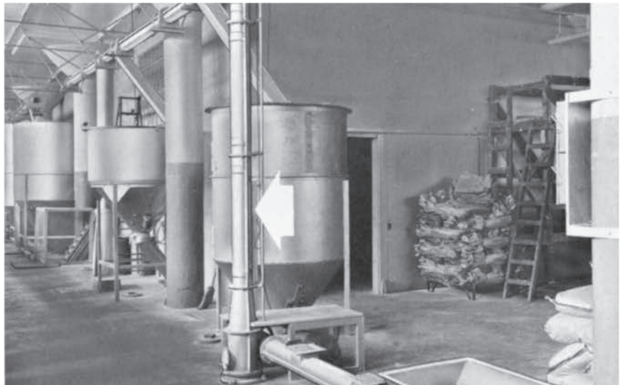
Screw-Lift and feeder moves material from floor to distributing conveyor over bins.
