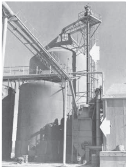
Outdoor installation shows two Screw-Lifts at large feed processing plant.
