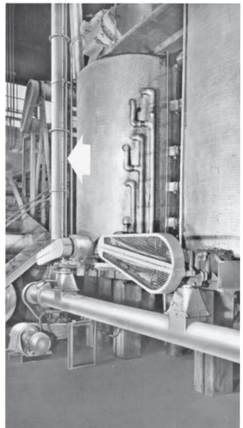
Installation illustrates Screw-Lift's compact arrangement with other equipment.
