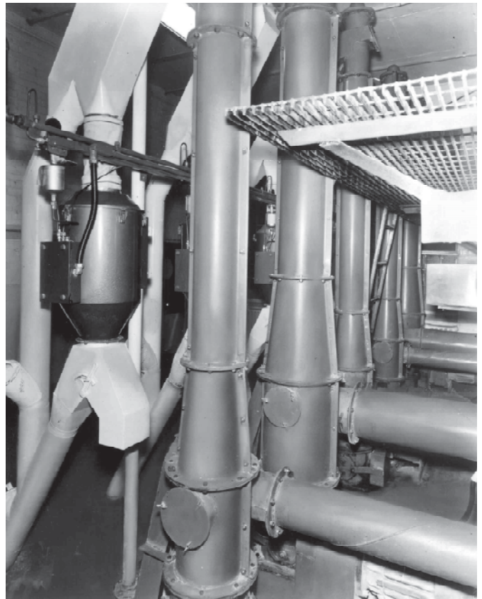
Rubber reclaiming operation uses high capacity, compact Screw-Lift and screw conveyor system to transport rubber back and forth between mills and screener.
