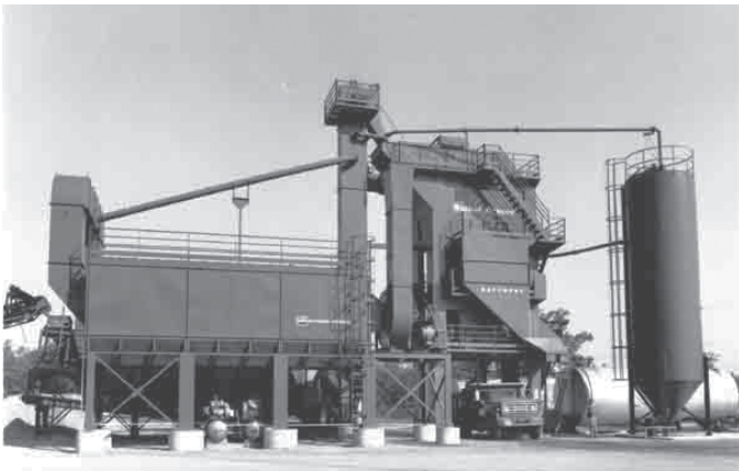
This asphalt fabric filter type dust collector uses Screw Conveyor flighting in the hoppers which return collected fines to the mix.
