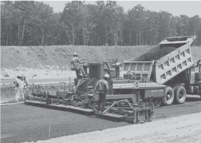
This Matmaker asphalt finisher uses a Screw Conveyor at the back of the tractor unit to move material outward in both directions and to spread it uniformly across the entire paving width.
